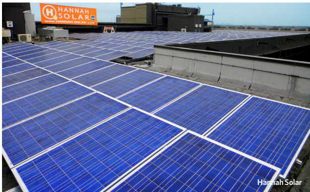
Solar array in Georgia built by Hannah Solar.
