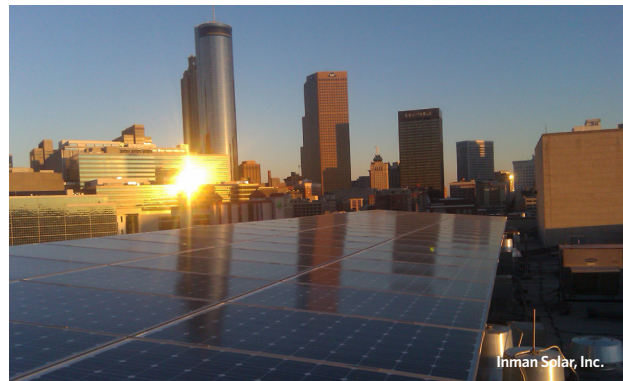
Solar array in Georgia built by Inman Solar.
