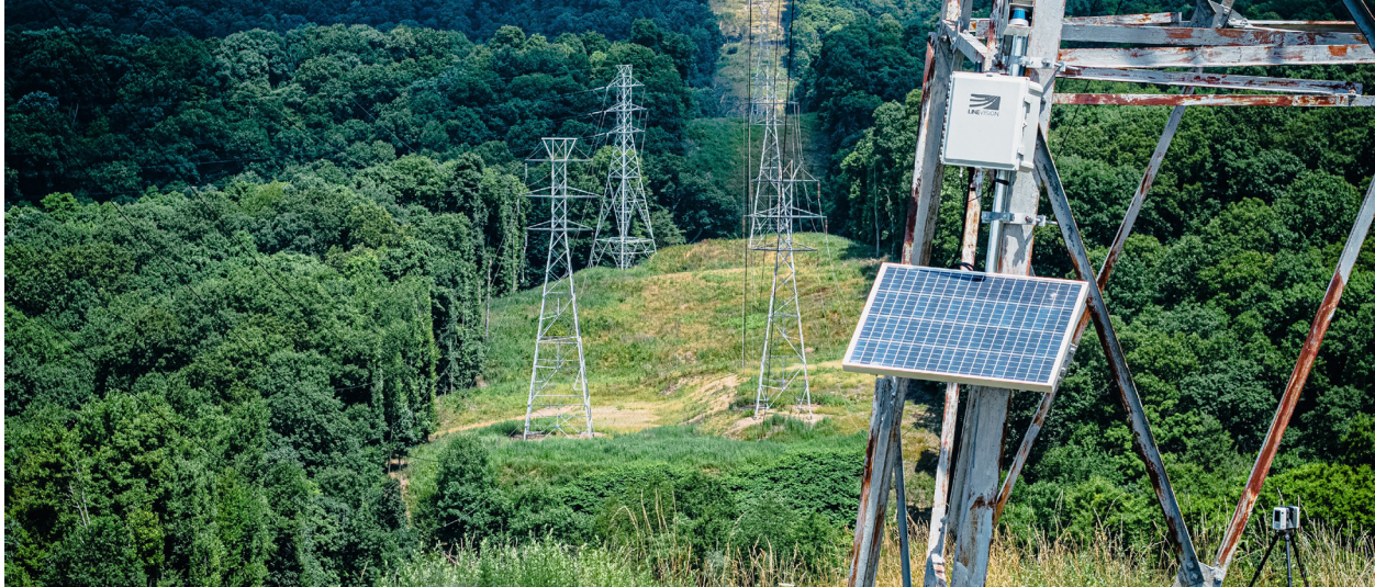
Dynamic line rating systems like this one collect critical transmission line information in real time to detect risks, assess conductor health, and enhance line capacity. LineVision
