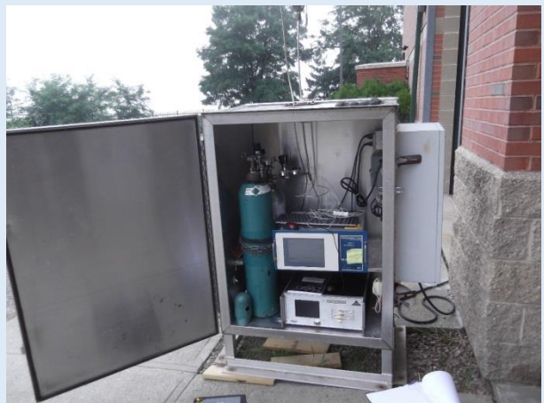
Mini-station at Weymouth MWRA Pump Station
